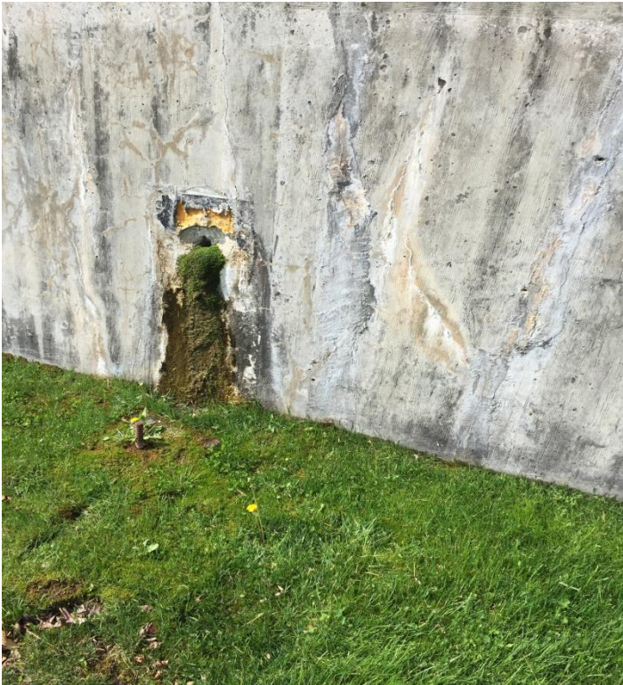
Failed tieback (note anchor plate and portion of tieback on ground)
