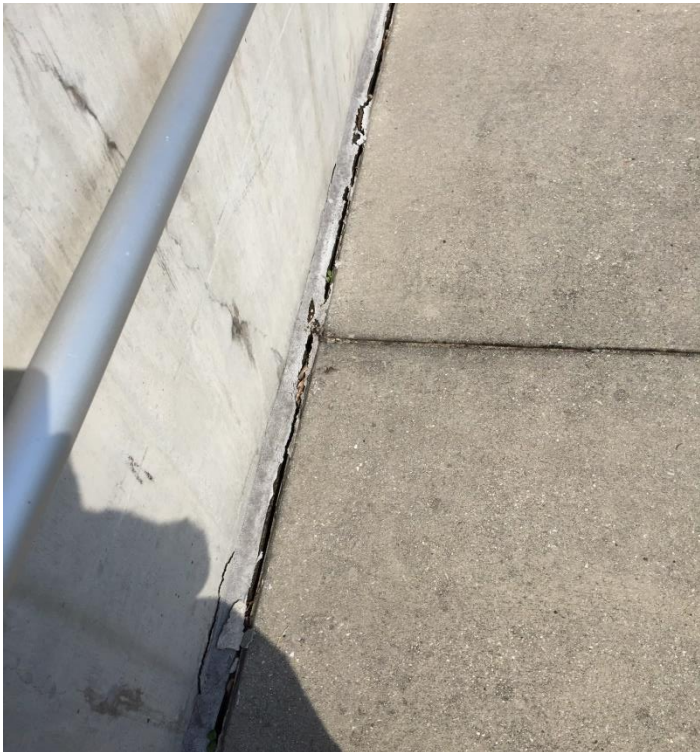
Failed joint sealant and gap between ramp and upper wall
