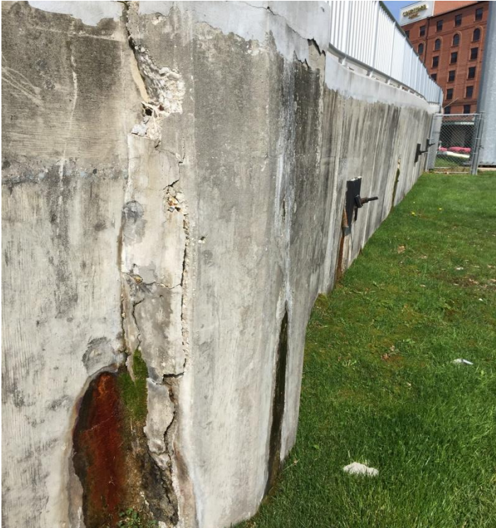
Cracks and spalls at pilaster
