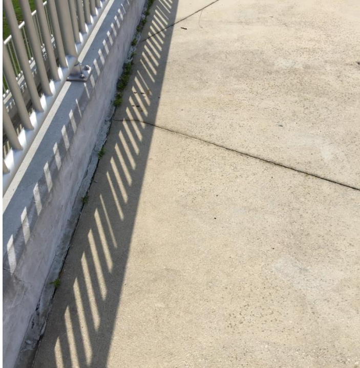
Failed joint sealant and gap between ramp and lower wall
