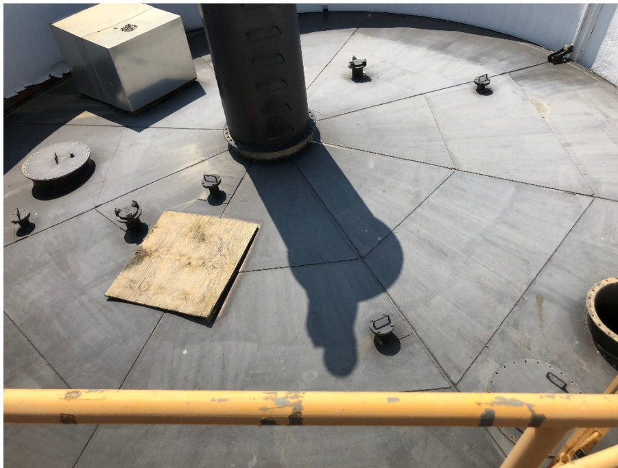
Digester #1 Cover top view
