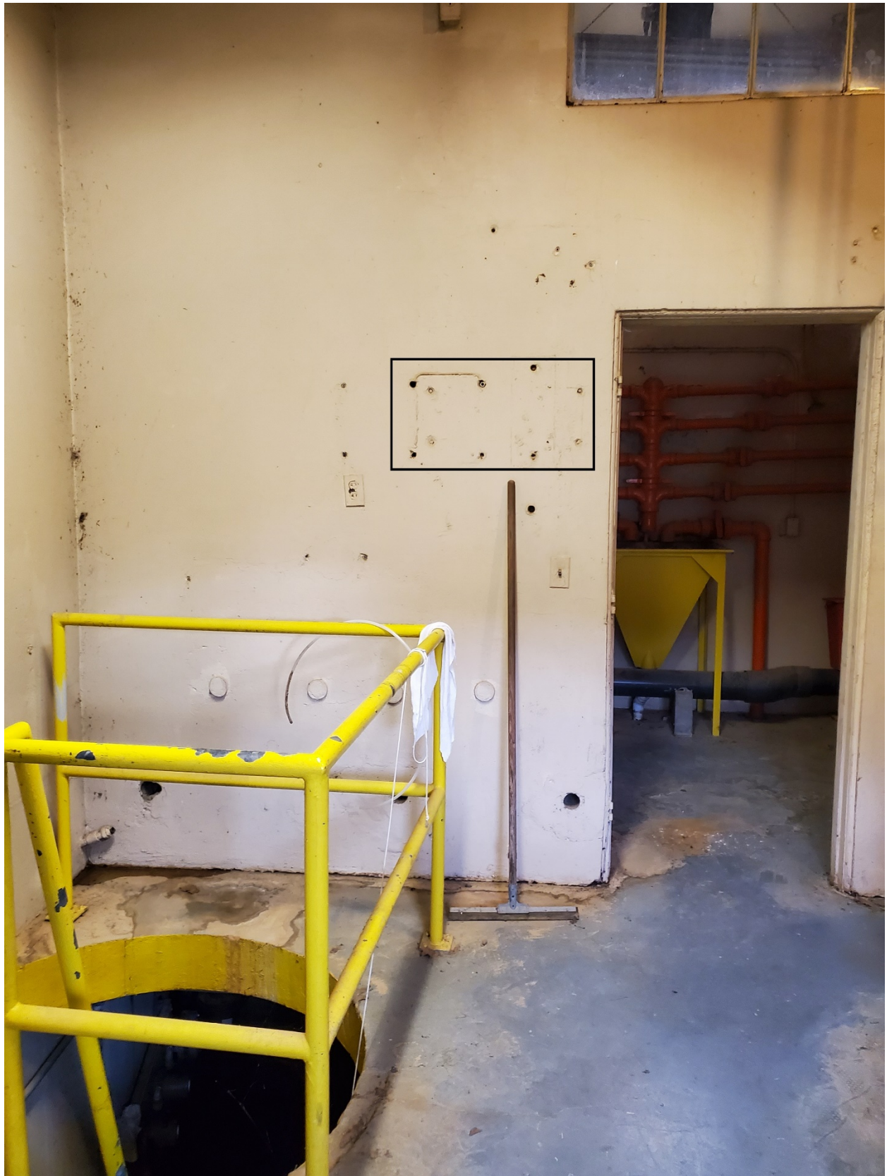
Interior of Digester Control Room – Location of Level Sensor Indicator Panels on Wall APG WWTP Digester 1 Cover Replacement Page-5 Addendum No. 1
