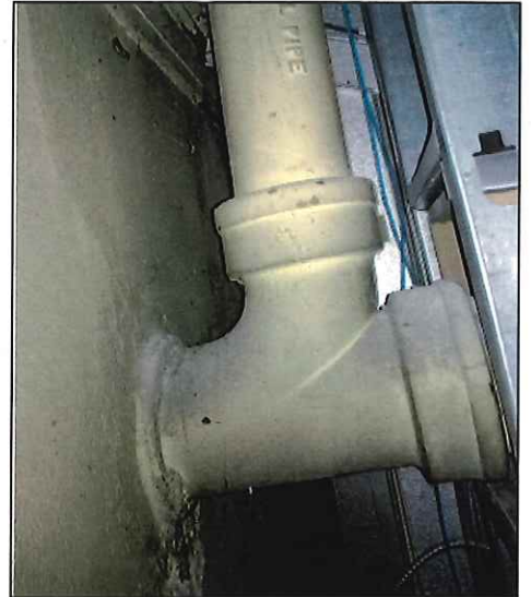
Sanitary Sewer Pipe
