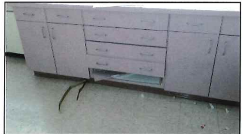
Worn Casework (2nd floor)
