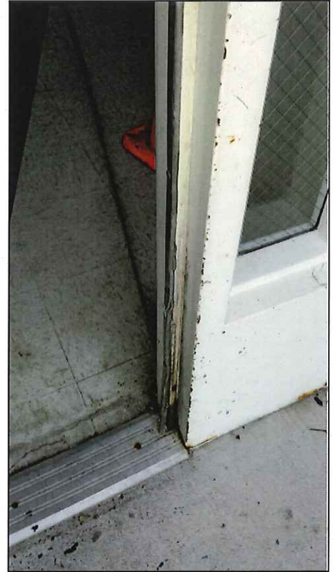
Damaged and Rusted Frame
