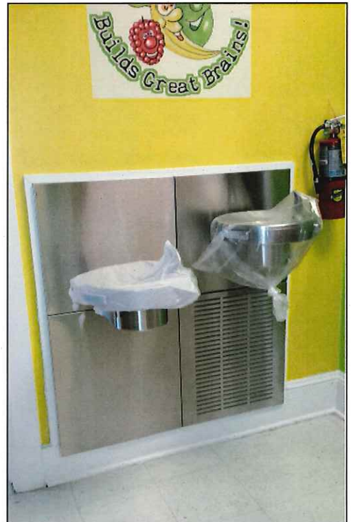
Only Compliant Drinking Fountain
