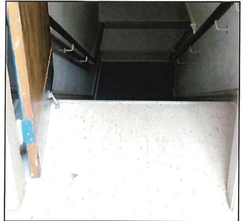
Non-Code Compliant Landing Size
