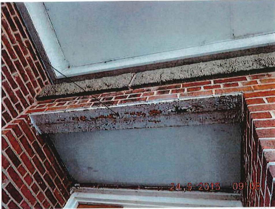
Photo 1 Exterior lintel on south side of rear by addition with lead paint in poor condition.
