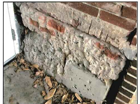
Exterior Degrading Brick and Attempted Repair
