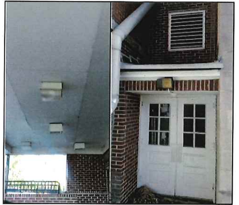
Exterior Lighting Fixtures
