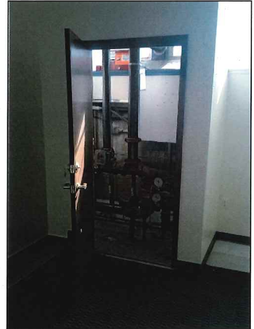
Fire Main - Entrance Point
