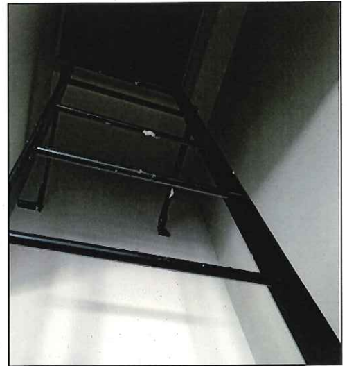
Ship's Ladder/Roof Access
