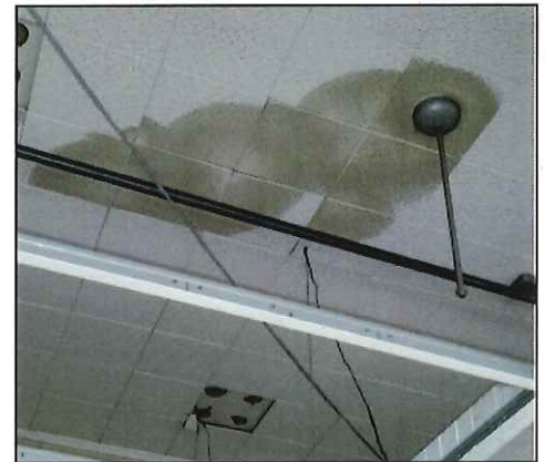
Water Damage and Falling Hard Ceiling
