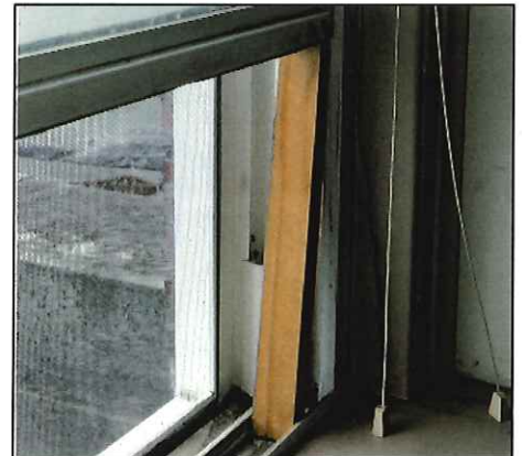
Inoperable Window Condition
