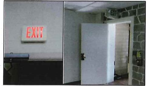
Ceiling and Wall-Mounted Exit Signs
