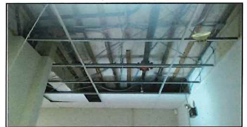
Sprinkler System Beyond Drop Ceiling
