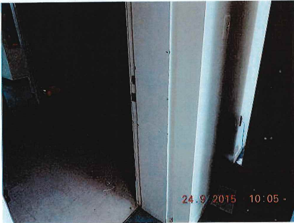
Photo 6 Lead paint on door trim, casings etc.
