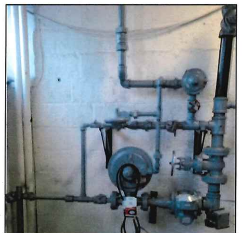
Natural Gas Regulator, Meter, and Piping
