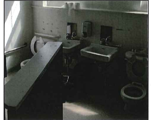
Children's Toilet Room
