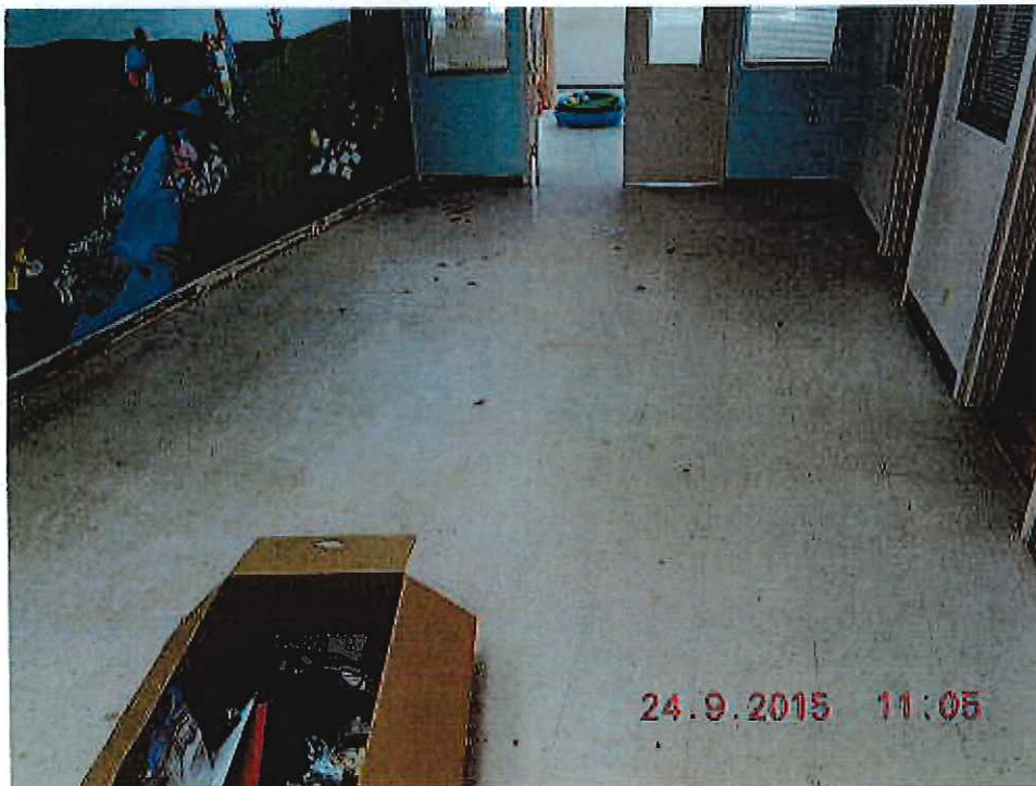
Photo 12 Much of this newer 12" floor tile is covering older 9" Vat/Mastic
