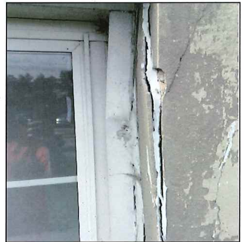
Exterior Lower Wall Crack/Parging and Attempted Repair
