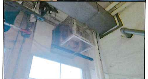
Boilers and Intake Fan
