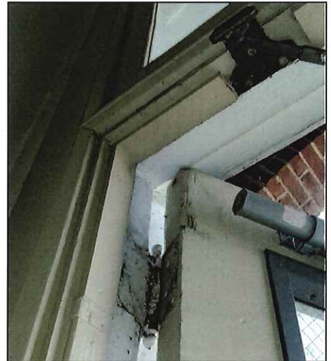
Damaged, Old and Rusted Hardware
