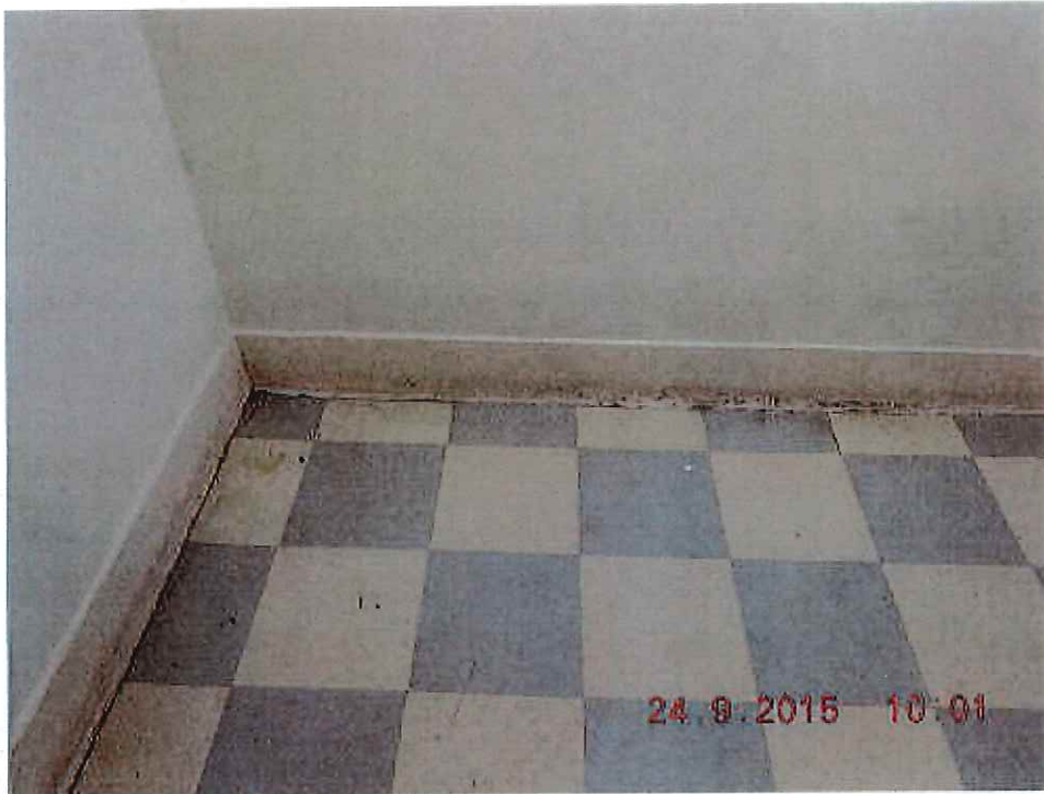
Photo 5 12" floor tile – negative. All 12" floor tiles were negative except those by the elevator lobby.
