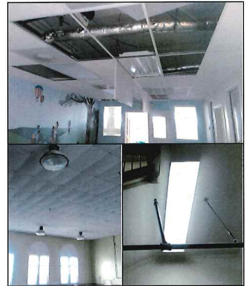
Interior Lighting Fixtures
