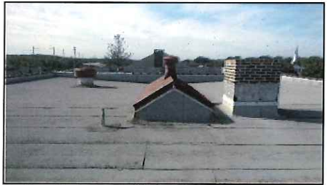
Boiler Exhaust Chimney
