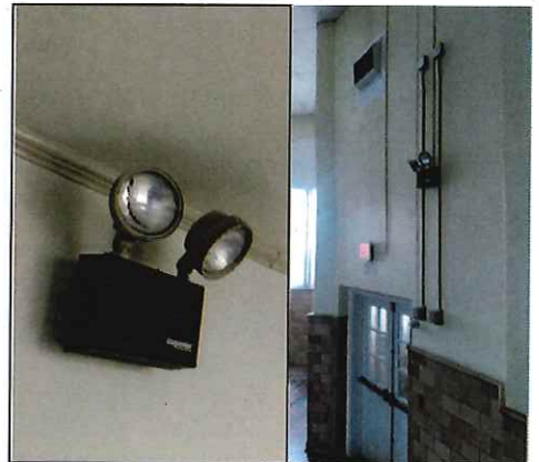
Emergency Lighting Fixtures
