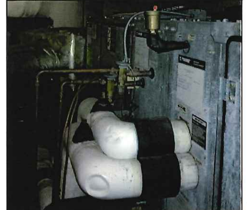
Constant Volume Air Handling Units
