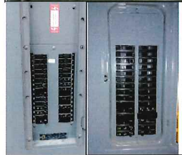
Panel Boards and Circuit Breakers
