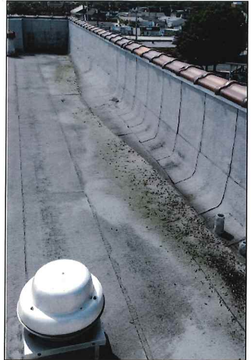
Stained Location from Ponding Water
