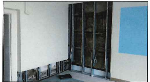
Children's Toilet Room
