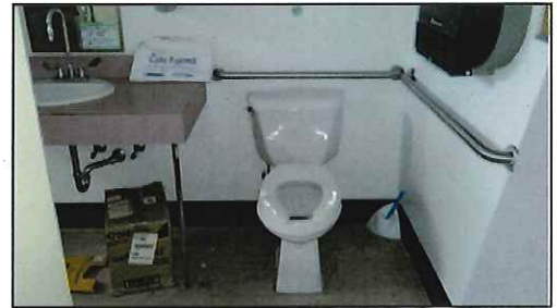
Non-Compliant Toilet Clearance
