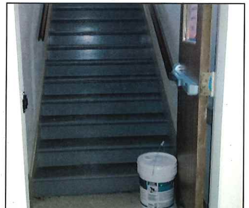
Non-Code Compliant Handrail, Landing, & Tread Material
