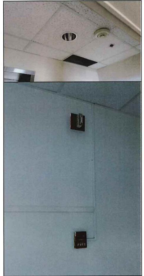
Fire Alarm System
