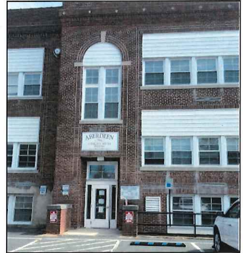
Weathered Brick Joints and Obvious Efflorescence
