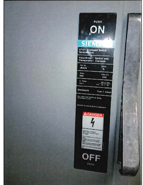
Elevator Controller, Panelboard and Disconnect
