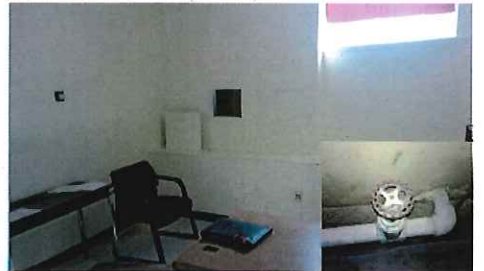
Water Service Entrance - Office 105
